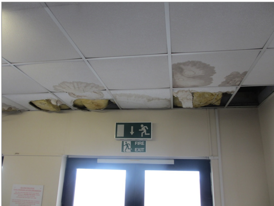
Figure 2: Evidence of water entering terminal building
